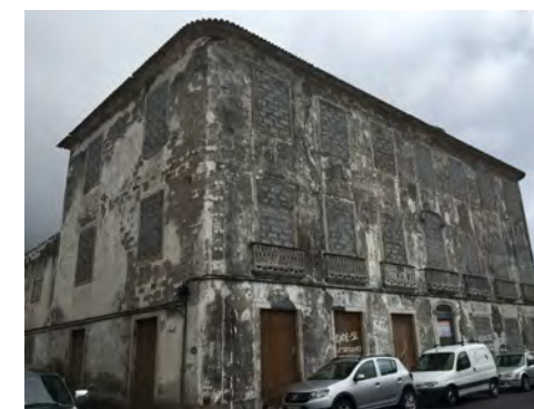
(Fig 4) Typical abandoned volcanic block apt building in the city center.
